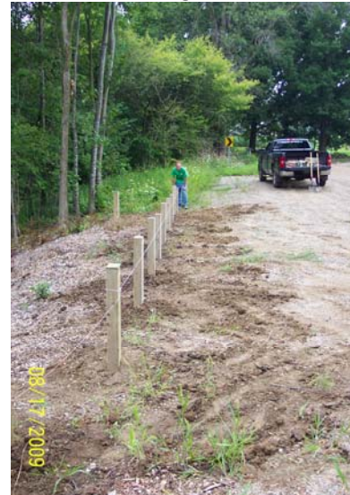
MSU Intern Eric Dobbrastine inspects alignment of posts at Maple River Public Access Site (French and St. Clair Roads).
