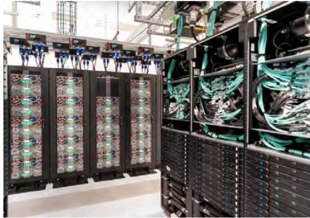
Water-cooled high computing systems in a data center. Credit: ECMWF Data Center.
