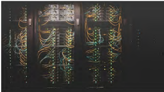
Fig. 1. A photograph of physical infrastructure essential for contemporary data management and storage in a modern data center. Photo by Taylor Vick on Unsplash (available for free use).
